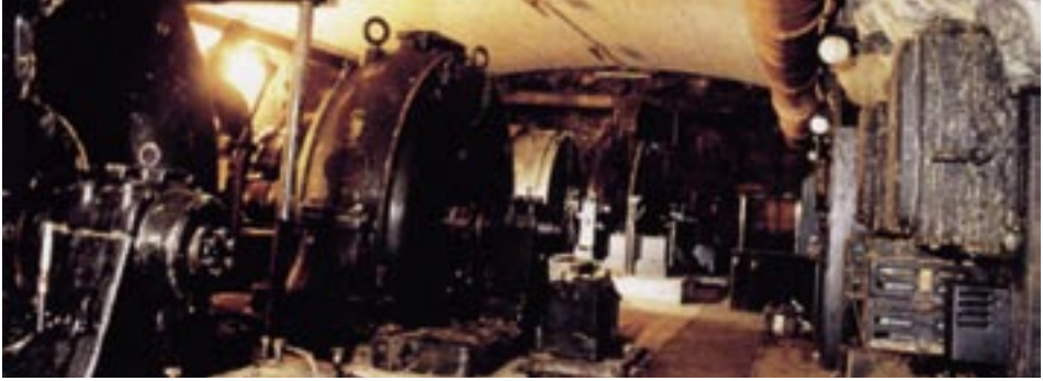
Underground electrical power station at the former "Drei-Brüder"-Mine in Freiberg (built 1913)
